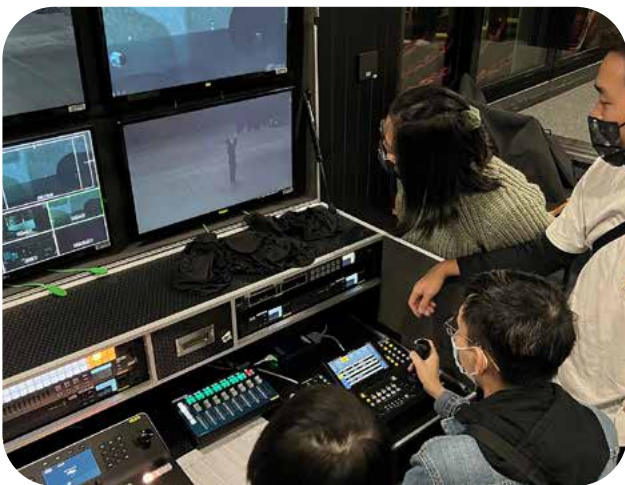
4K remote-controlled cameras and live streaming systems have been installed in the Kwai Tsing Theatre and Tsuen Wan Town Hall, enabling online programmes to be presented in 4K resolution and performing groups to create multi-angle 4K archives.
