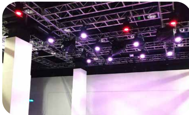
Computerised moving lights have been installed in the Cultural Activities Hall at the Ngau Chi Wan Civic Centre to enhance the venue's technical capabilities.
