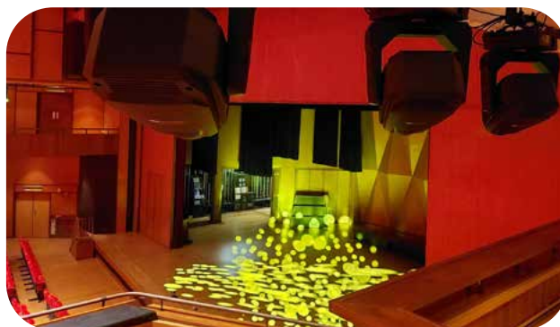
LED moving lights and LED profile spotlights have been installed at the Auditorium of the Tsuen Wan Town Hall to give lighting designers more creative design options.
